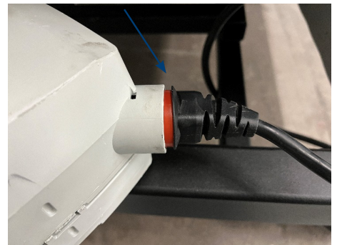
Disconnected power cord
