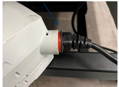
Disconnected power cord
